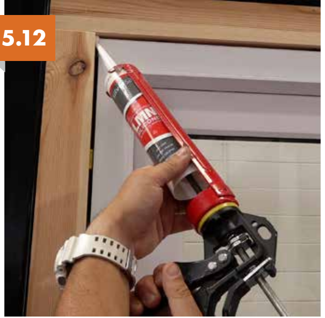
Silicone sealant using a low modulus sealant to finish around the frame.
